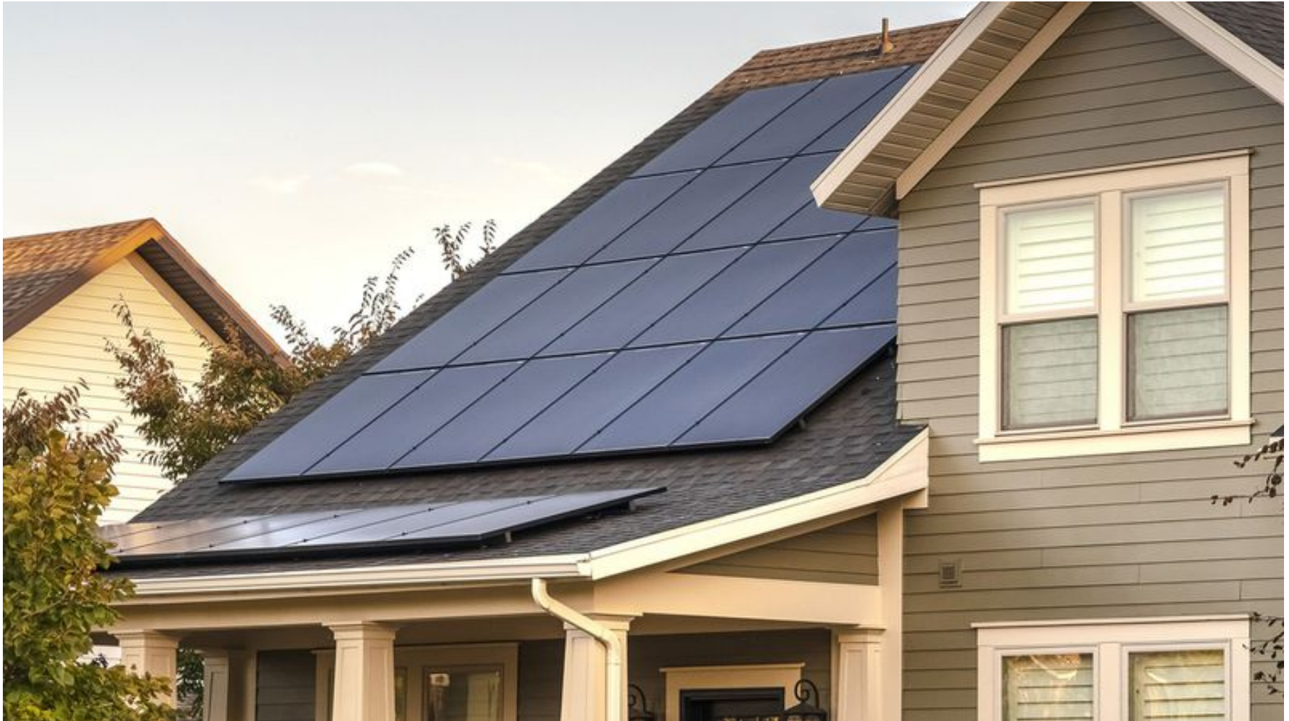
Solar panels on a home. As natural gas costs rise, electrification can present a more affordable option, especially with growing sources of renewable energy like solar. (Dreamstime)
